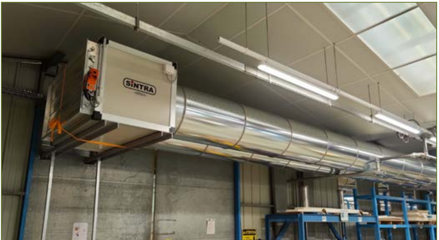
- REVERSIBLE AIR CONDITIONING
